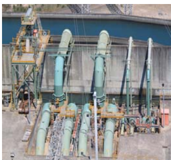
Condenser system at Eraring Power Station
